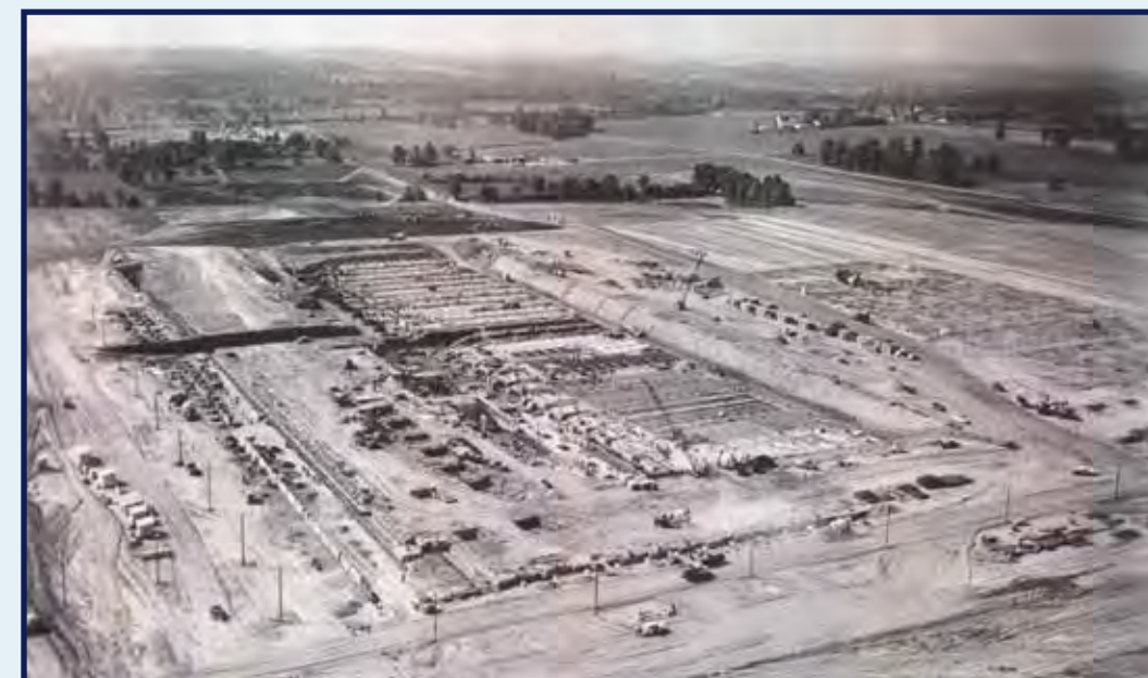
The General Motors Fisher Body Stamping Plant under construction in 1956. Photo courtesy of the John Sherman Room, Mansfield/Richland County Public Library.
