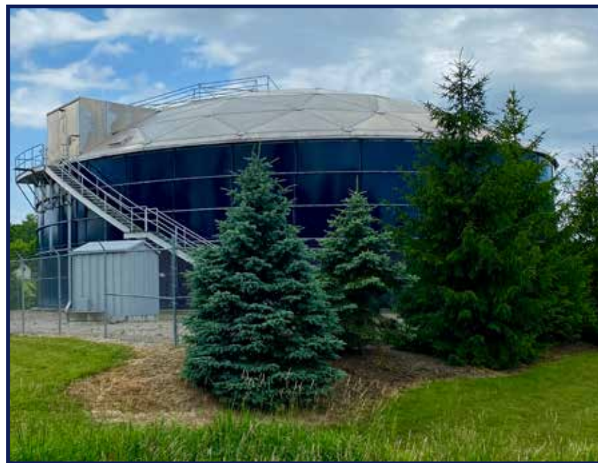
An above-grade flow equalization basin at Rock Road.
