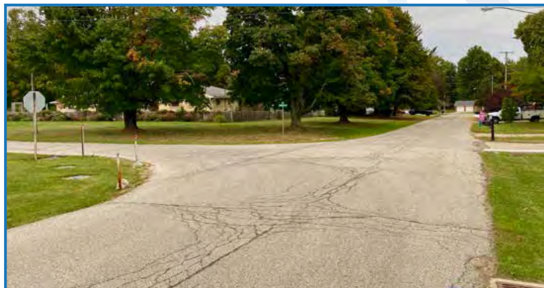
Inflow & Infiltration (I&I) occurs throughout the community, particularly in uncurbed neighborhoods.
